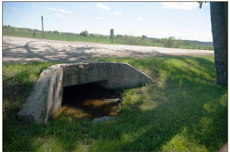
Undersized and eroding culverts contribute to flooding when water backs up during storm events, especially on flat agricultural lands. (Photo by Headwaters Economics)
